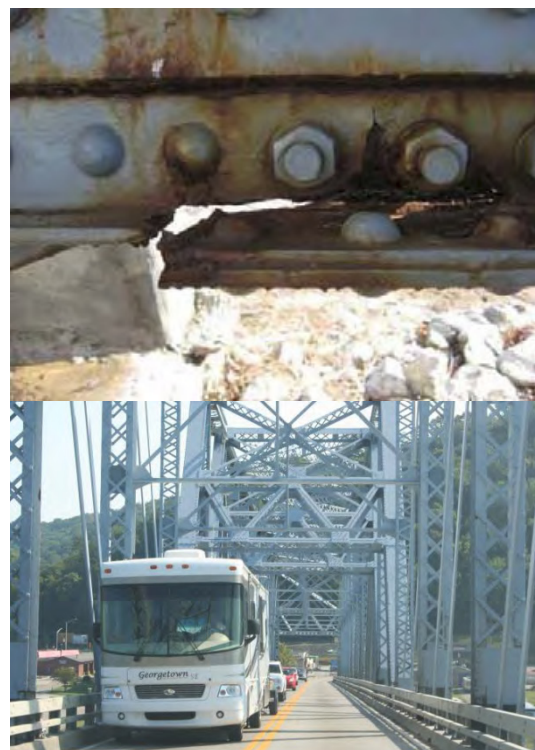
Structural damage was one of the many reasons KYTC and INDOT moved forward with the bridge replacement (top). The old bridge's 20-foot-wide road deck could not accommodate commercial traffic and the bridge had a weight limit of 3 tons (bottom). (Courtesy of FHWA Indiana Division Office)
