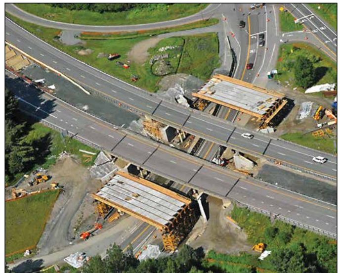
Vermont Agency of Transportation (VTTrans) Accelerated Bridge Program. Image courtesy of VTTrans.
