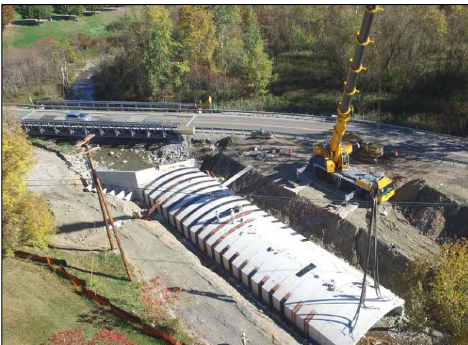
Duxbury Culvert Replacement that benefited from Expediting Project Delivery . Image courtesy of VTrans.
