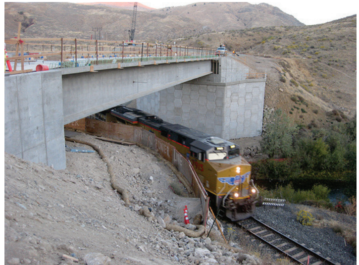
A train passes through a construction worksite within the right-of-way. (Courtesy of FHWA)
