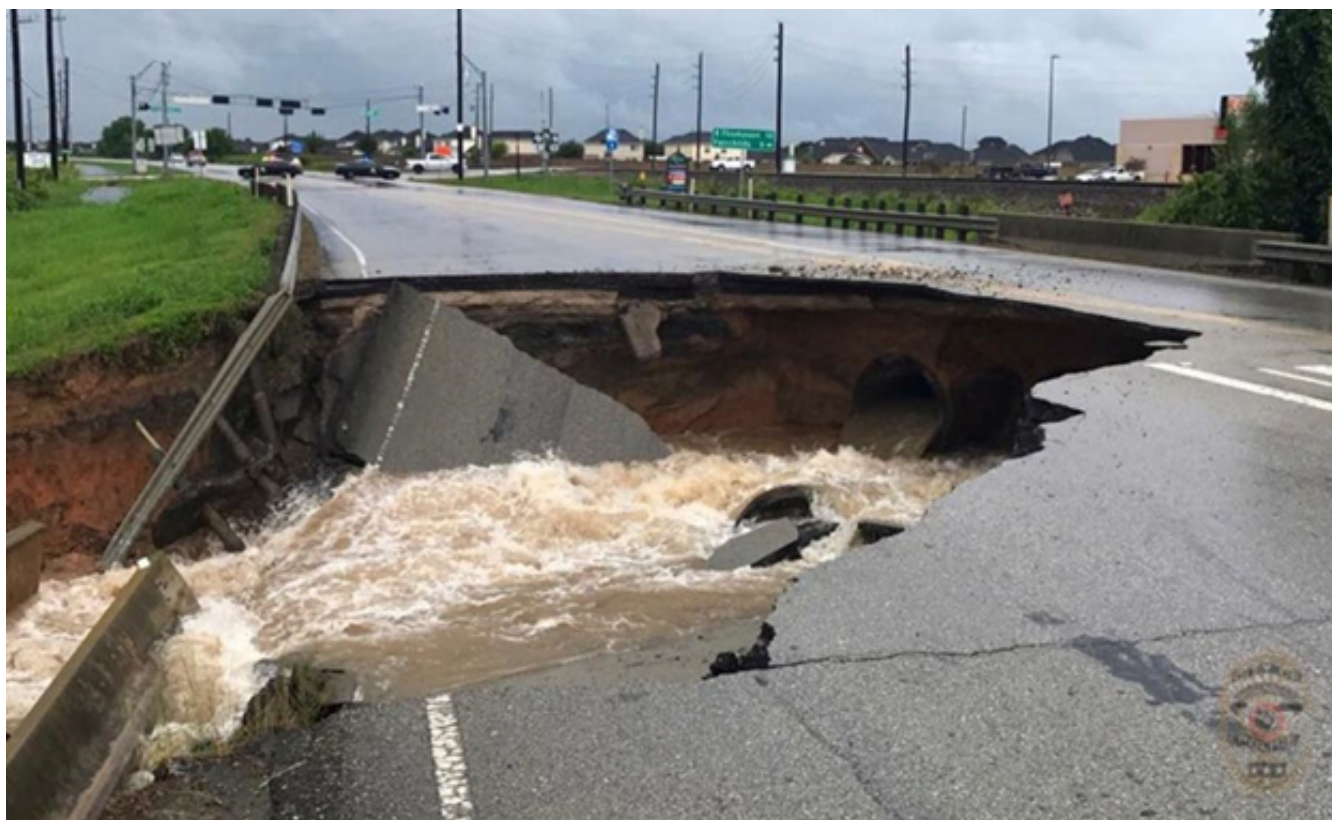
Hurricane Harvey Damage, 2017; Houston, TX. Image courtesy of Engineering News Record .
