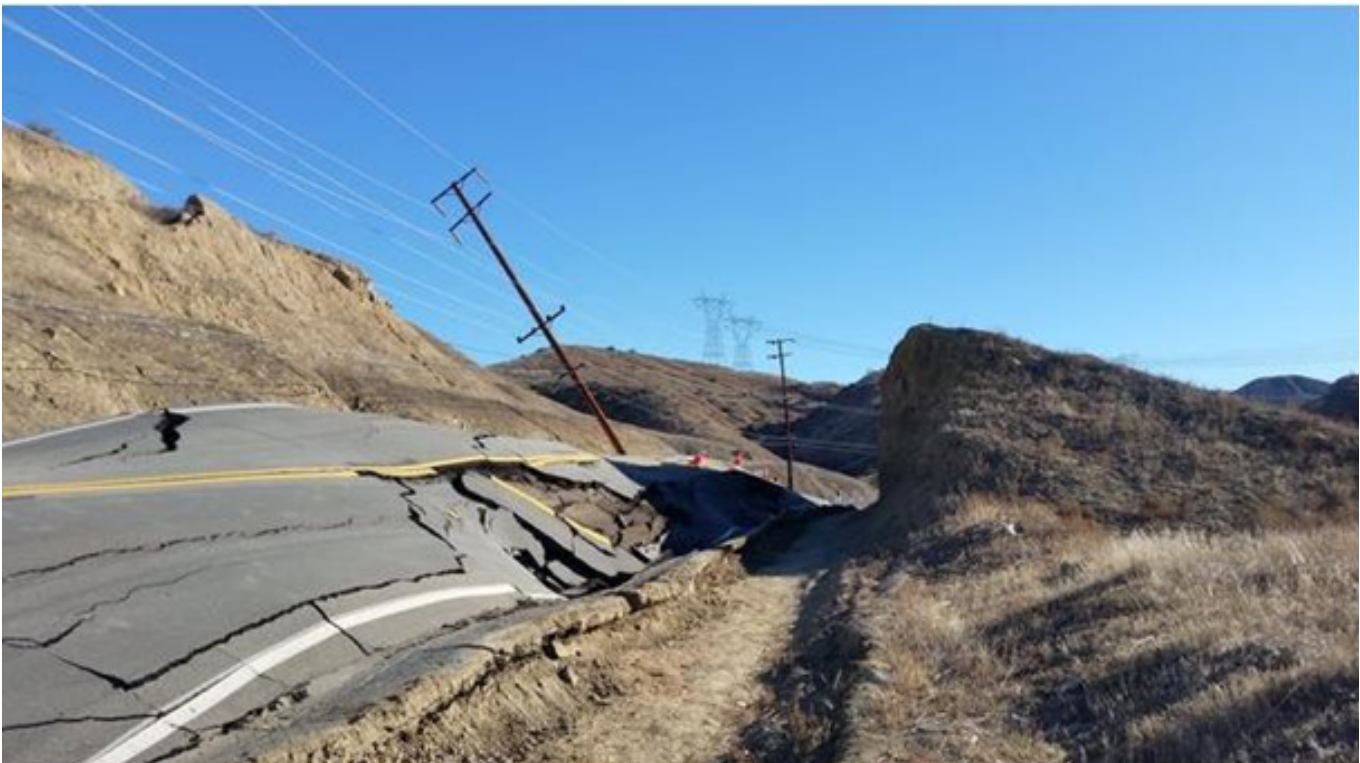
Damage from a landslide in 2015; Santa Clarita, CA. Image courtesy of SFGATE .
