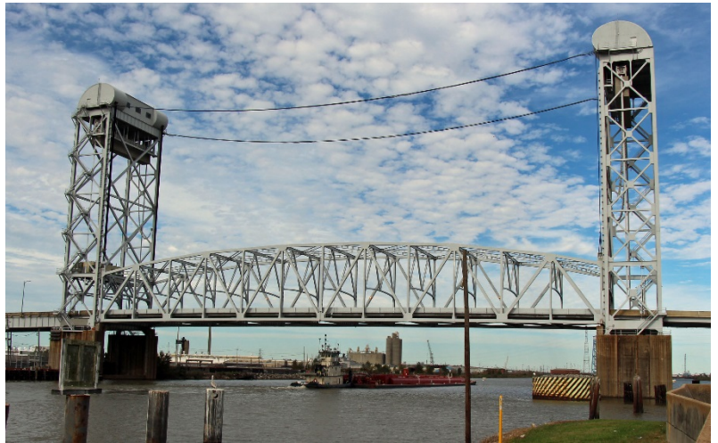
The State Route 39 Inner Harbor Navigation Canal Bridge, also known as the Judge Seeber or Claiborne Avenue Bridge—built in 1957—has a steel vertical lift span. It was labeled a “Preservation Priority” bridge and was recently rehabilitated. (courtesy of LADOTD)
