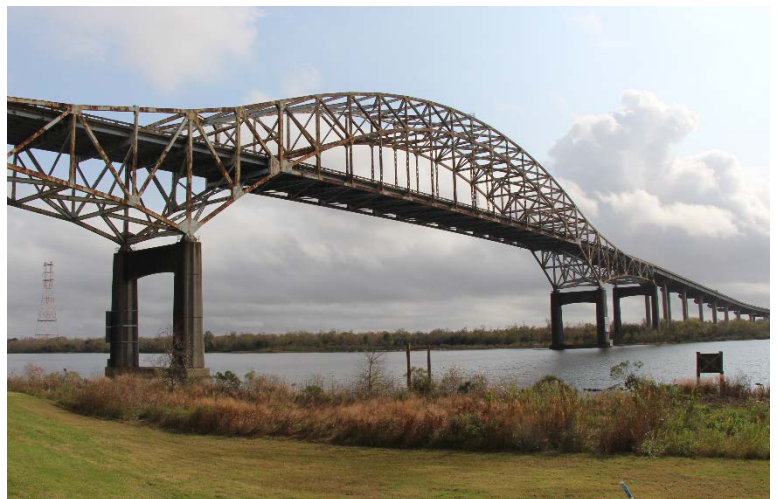
A rehabilitation project is scheduled for the Gulf Outlet Bridge, a "Preservation Priority" bridge. (courtesy of LADOTD)
