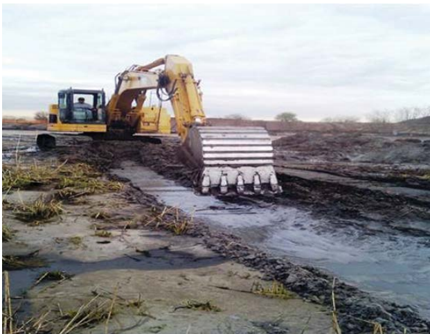
Workers begin construction of a wetland restoration project at Gerritsen Creek in Brooklyn. (Courtesy of New York City Department of Parks and Recreation)
