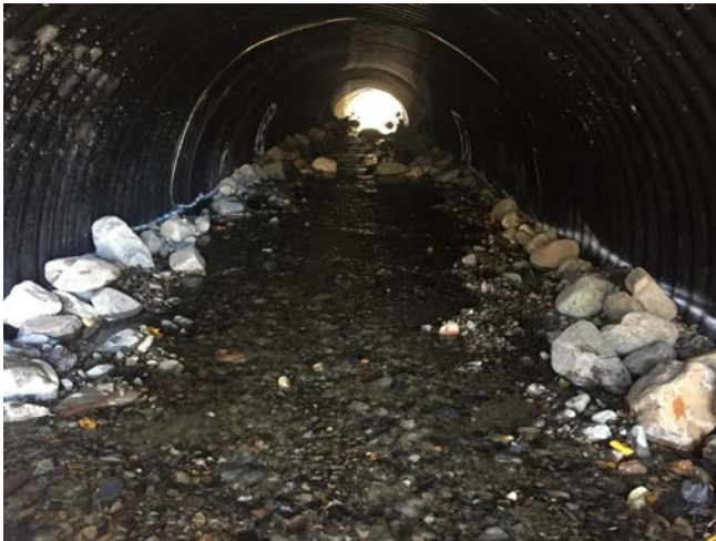
Completed culver replacement at Dyer Brook, ME using stream simulation methods (Courtesy of MaineDOT)
