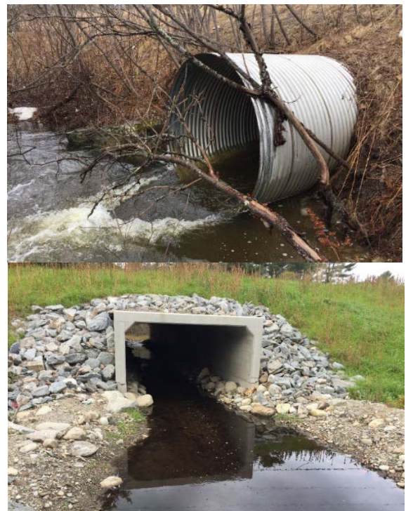
Before (top) and after (bottom) Route 139 Winterport Culvert Replacement (Courtesy of MaineDOT)
