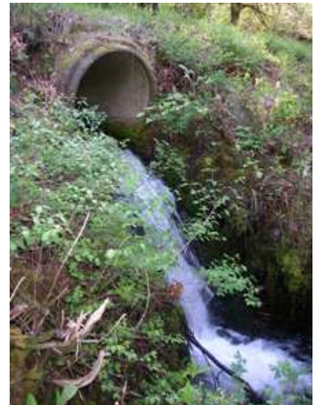
This culvert is a barrier to fish passage because its opening is too high for fish to jump into, preventing them from reaching their upstream habitat. (Courtesy of WSDOT)
