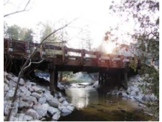
A 30-foot timber bridge replaced the culverts that once spanned the Black River. (Courtesy of USFWS)
