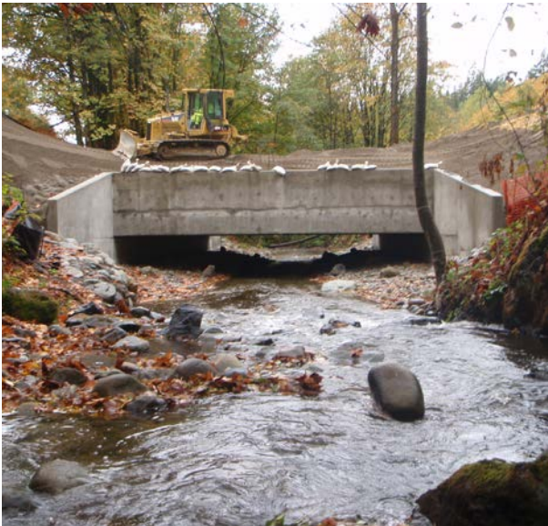
Natural streambed material underneath the East Fork Issaquah Creek culvert simulates nearby stream conditions. (Courtesy of WSDOT)
