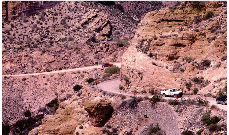
A road crew works near a historical stone wall on the Apache Trail in the Tonto National Forest. (Courtesy of USFS)
