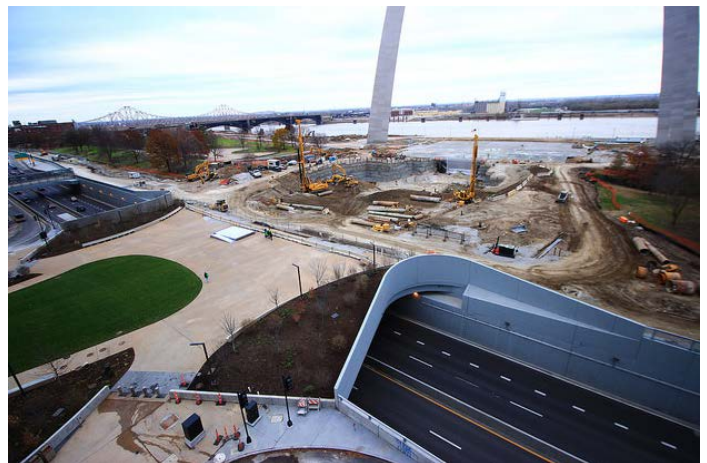
Completed freeway cap and Arch park grounds construction (courtesy of CityArchRiver Foundation)
